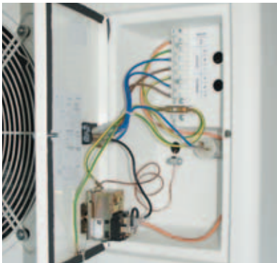
Convenient access to electrics for installation and maintenance
